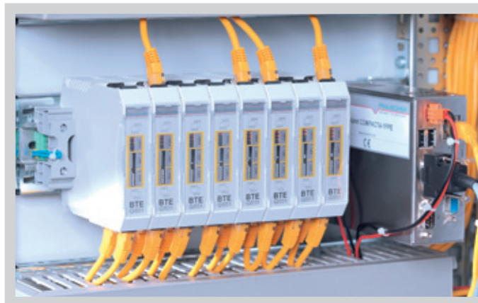
Figure 2: Bus transfer entity – BTE – Combined LOG processor and CAN bus
